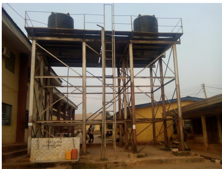
Figure 2: OVER-HEAD TANK AT THE TEMPOARY SITE
