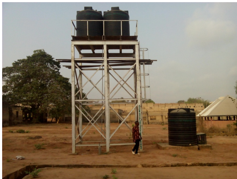
Figure 4: OVER-HEAD TANK AT PERM. SITE
