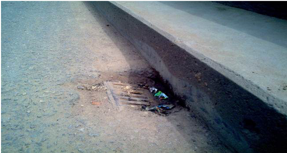
Figure 11. Poor Maintenance – Failure on edge of the pavement around gully.
