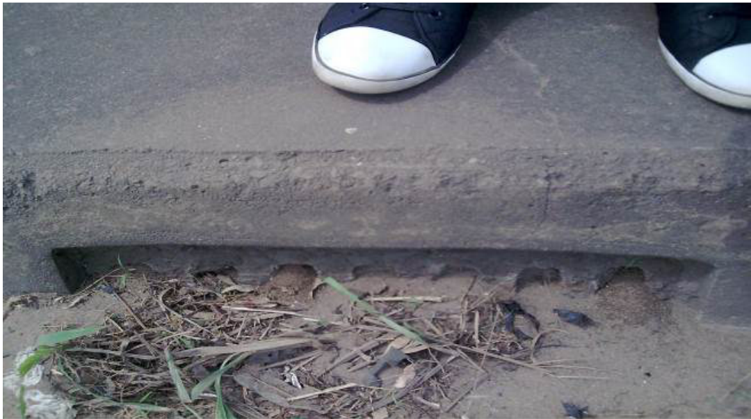
Figure 9. Poor Maintenance – Grating blocked with dirt, weed and Silt sand accumulation over time.
