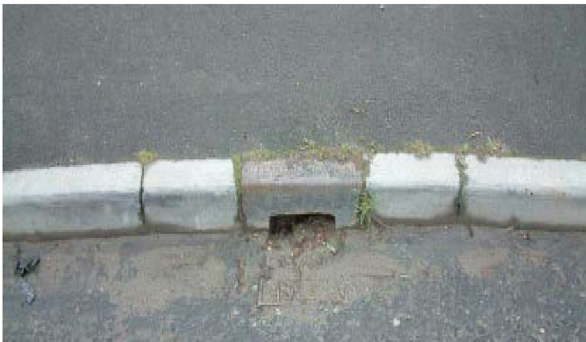
Figure 4. Poor Maintenance – Grating is barely visible.
