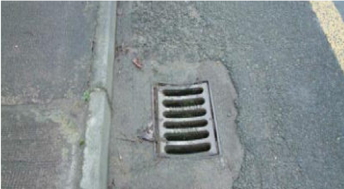
Figure 3. Gully is too far from kerb.
