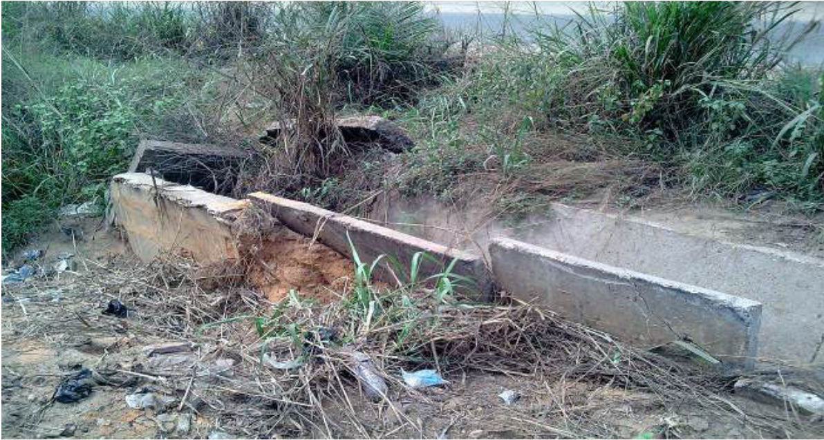
Figure 7. Failed Side drains overtaken with vegetation.
