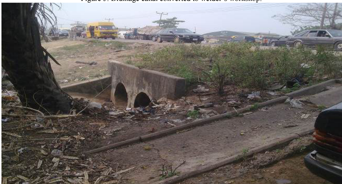
Figure 6. Culvert discharge points blocked with refuse dumps.
