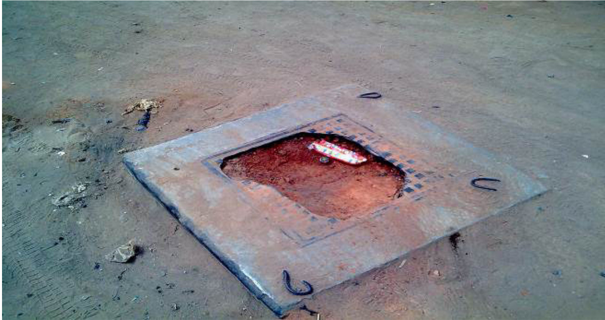
Figure 8. Poor Maintenance – Totally blocked underground drainage network.
