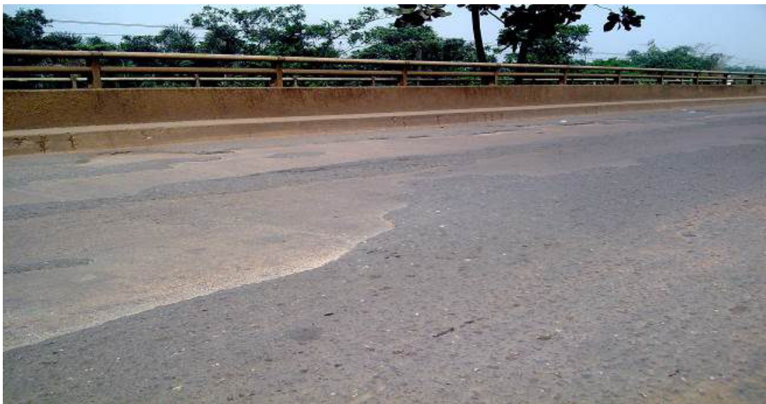
Figure 10. Detachment of bituminous pavement layer (stripping of bitumen).
